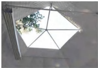
Auto Skylight Curtain
